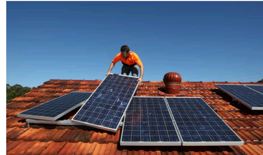
▲ Solar panels are installed on to the roof of a house in Sydney, Australia. Almost 90% of new electricity generation in 2020 will be renewable, the IEA says. Photograph: Reuters
